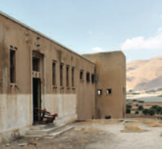
Fig. 50 Current condition of the old Prison in Jiftlic / Jiftlic’deki Eski Hapishane’nin mevcut hali
